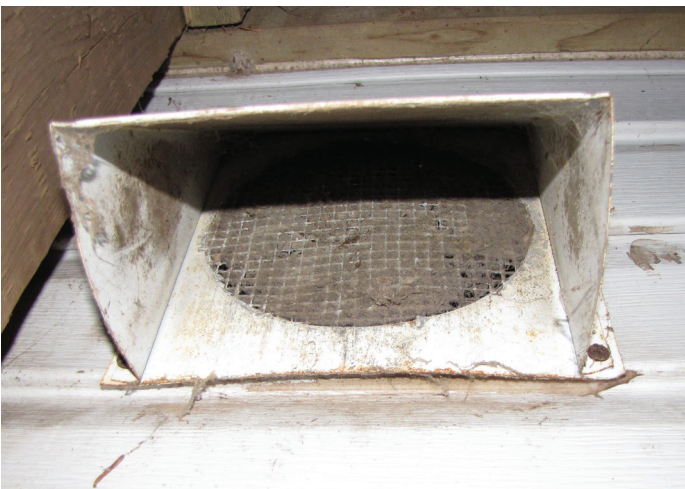
A poorly located air intake can collect debris and reduce performance and air quality.
